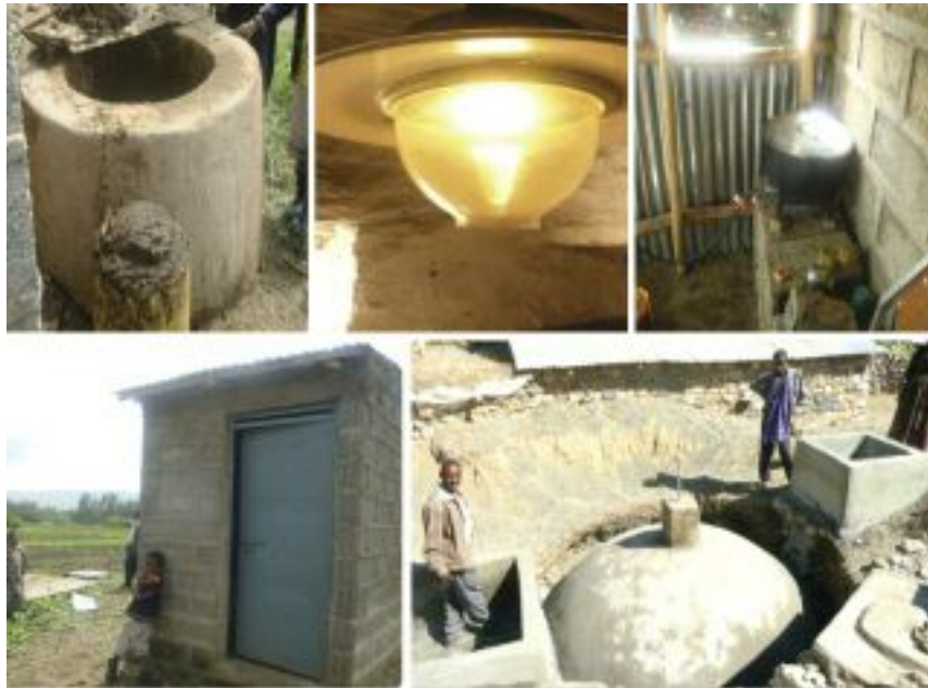
The construction of one of the biogas digesters which is linked to new pit latrines; the nuns now use biogas for cooking and electricity
