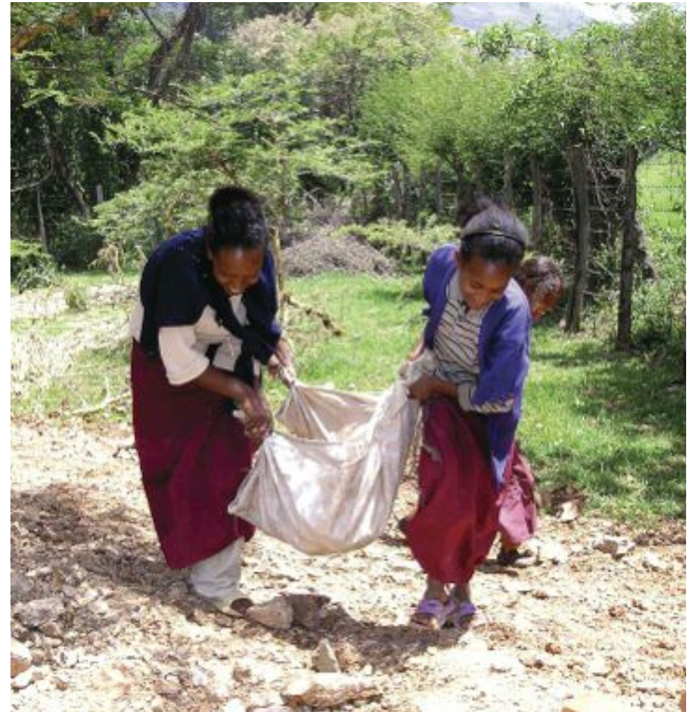
Pupils from the Junior Secondary School at the Sebata nunnery help in the construction of the biogas digester.
